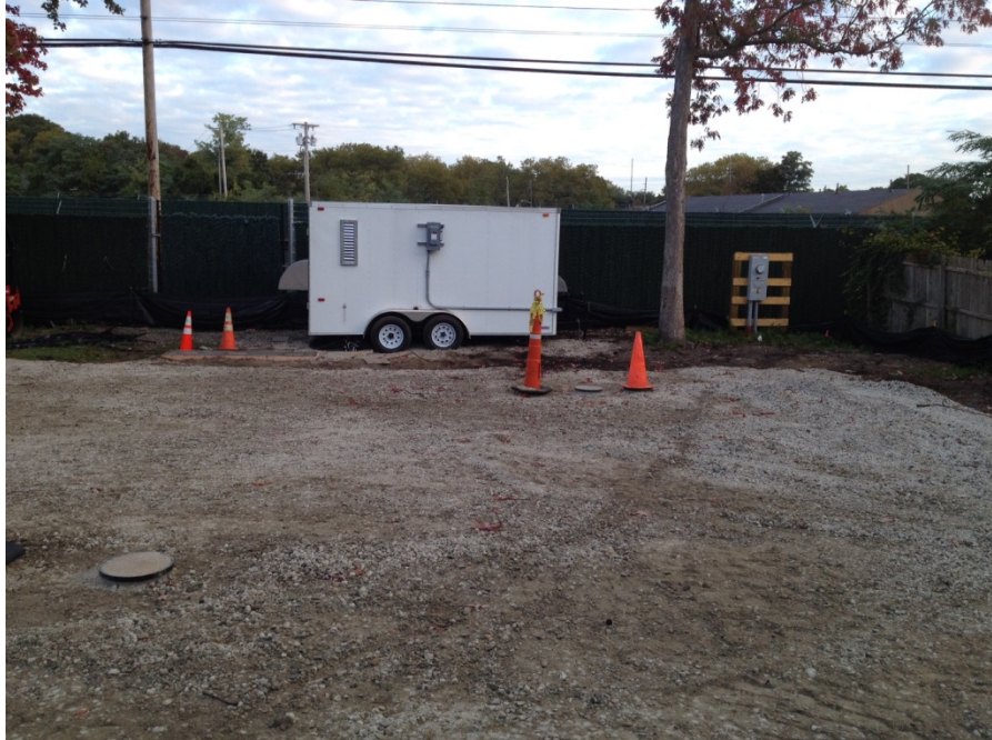
87 Community Road oxygen injection system location
